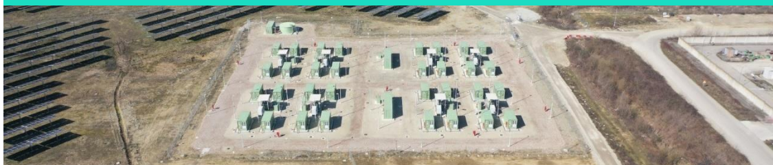
Image: Enel Libra Flexsys, Italian battery storage and open cycle gas turbines project
