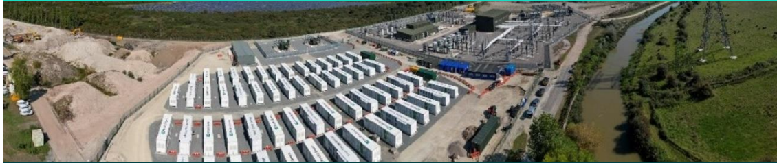
Image: Richborough Energy Park, UK battery storage project
